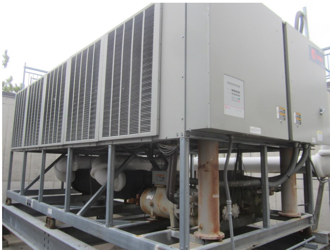
Figure 2. Air Cooled Chiller
